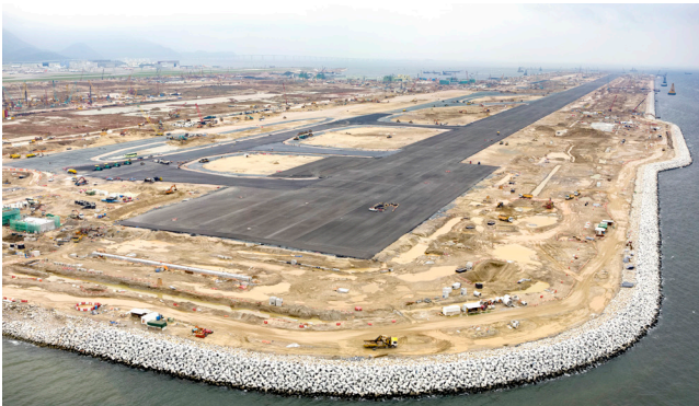
Completion of pavement works of the Third Runway (Photo courtesy of Airport Authority Hong Kong)
